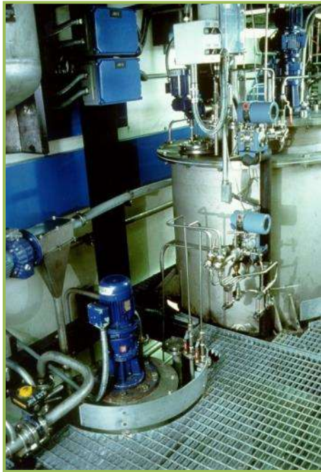
Chemical – Physical Treatment Flocculation section
