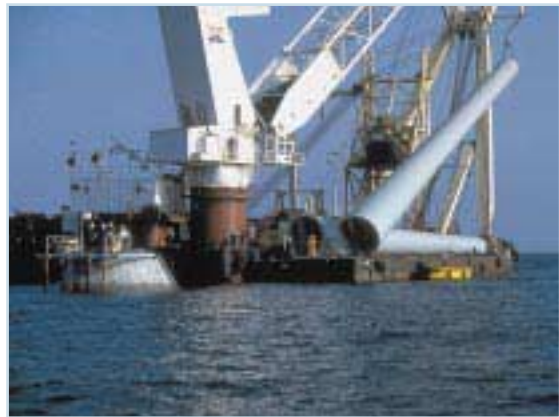
Figure 6.2: Tunø Knob offshore wind farm
