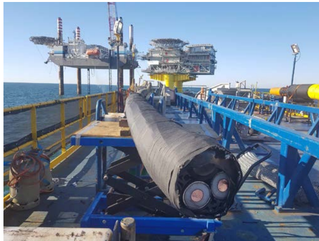
Cable Pull-in at OSS KFBE (Energinet, DK) One of the two sea cables during installation campaign in front of KFBE platform
