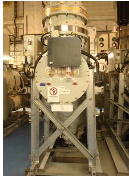
150-kV GIS 1 of 2 Reserve switch bays, 2015
