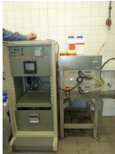
Figure 30. On-line river water radioactivity monitor
