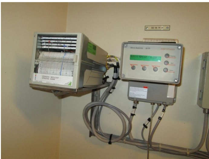
Figure 4. Kr-85 monitor of the aerial discharge monitoring system
