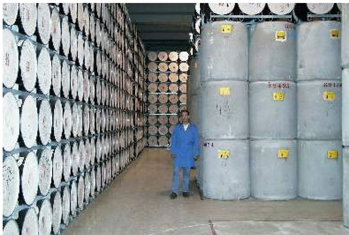
Figure A 3: Facility for interim storage of conditioned low- and intermediate level radioactive waste at COVRA
