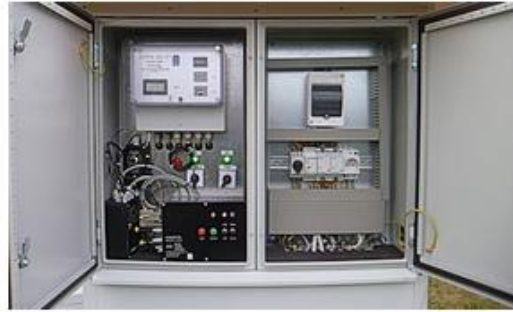
Measurement- and Power-Supply-Box
