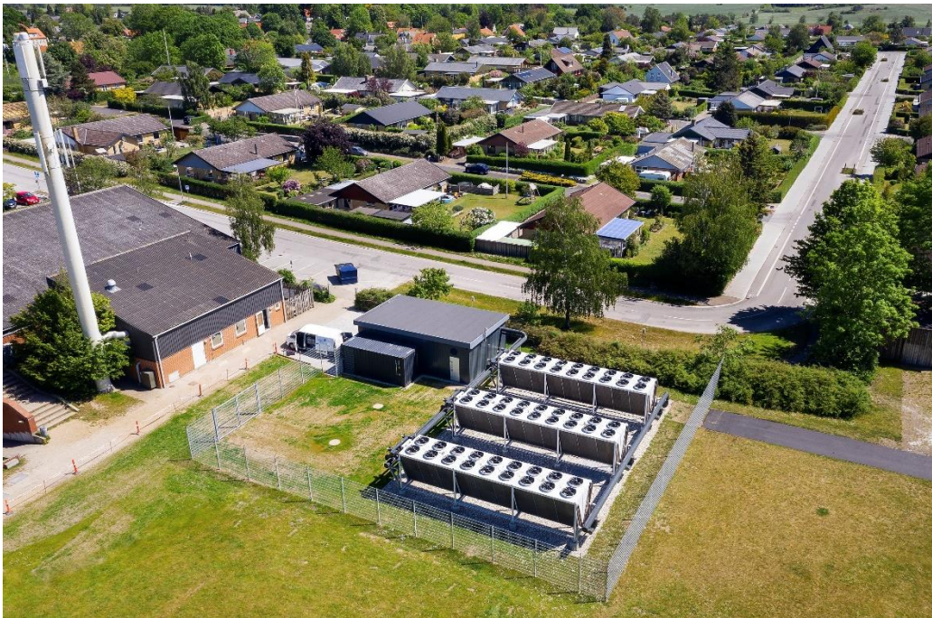
Figure 16: 1-MW air-source heat pump with air as the heat source, in Slagslund, Denmark (Courtesy of PlanEnergi)
