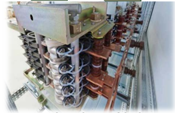
Picture: EONERC: ABB IGBT Stack
