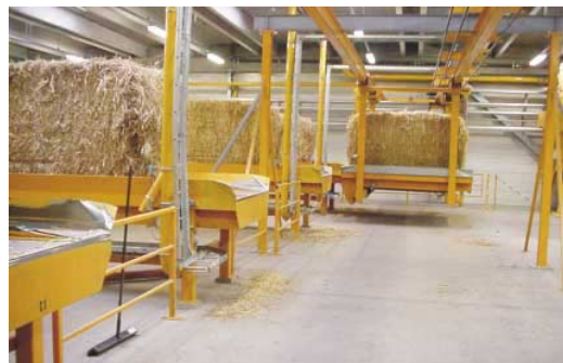
Straw is co-fired with coal in Denmark. DTI.
