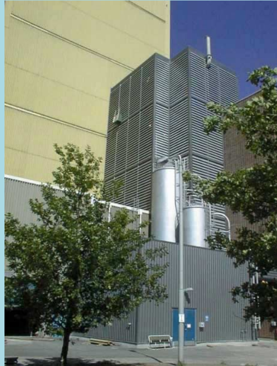
The Lahti CFB gasifier which is connected into 350 MW pulverised coal fired boiler has been in operation since 1998. Lahti Energia.
