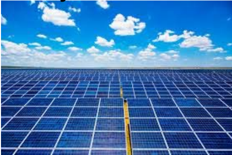
Utility scale PV
