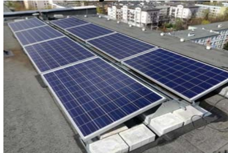
Community solar solutions
