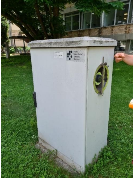
Figure 35. Single-branch high flow-rate air sampler at the JSI
