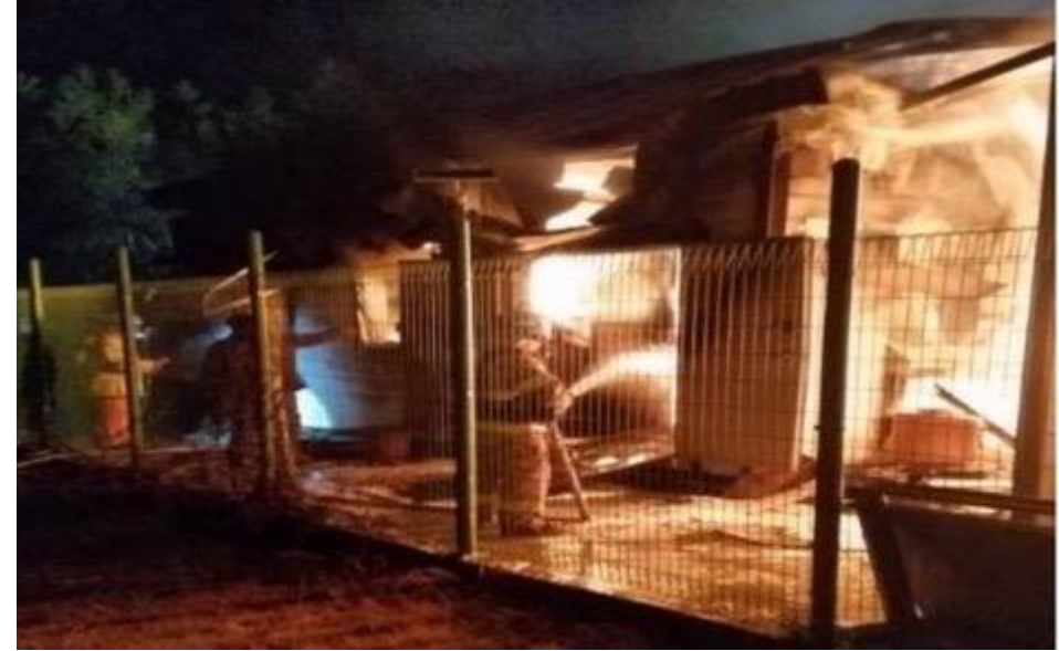
Samcheok PV power plant (Dec 2018, Korea)
