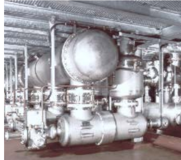
1968: First 170 kV GIS (SF 6 ), Zürich, Switzerland
