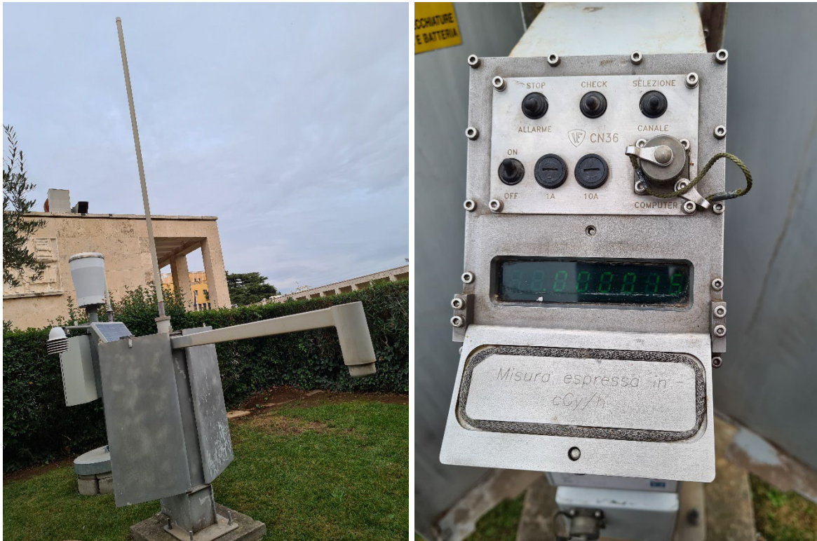
Figure 23. XR-33 automatic fallout radiation monitoring station with a local display at the CNVVF centre
