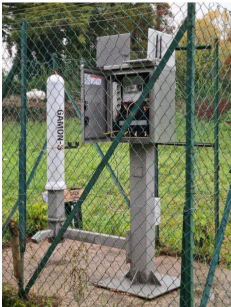
Figure 3. GAMMA network automatic monitoring station
