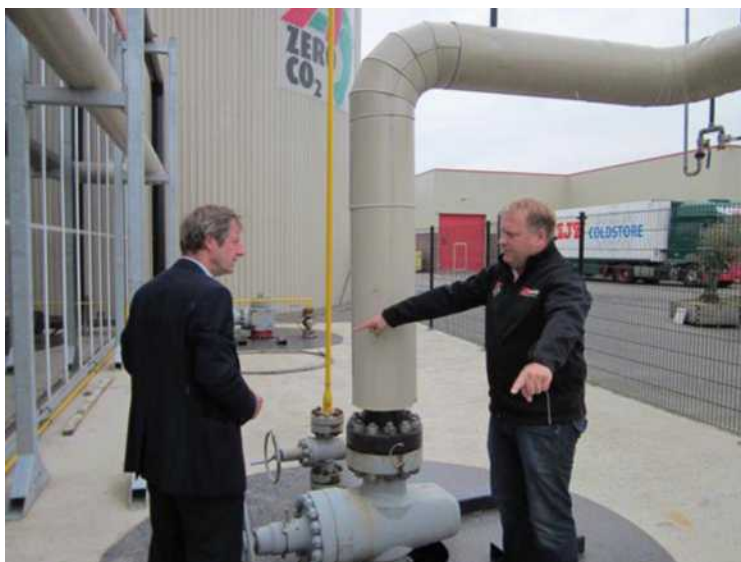
Figure 16 Geothermal energy plant at Ammerlaan in Pijnacker
