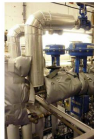
Steam valve insulation
