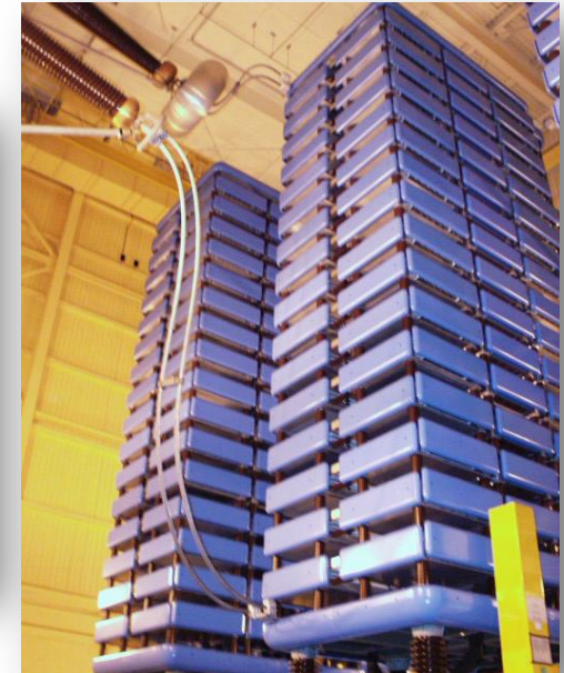
Thyristor towers: 96 thyristors 250 KV – 2000 A
