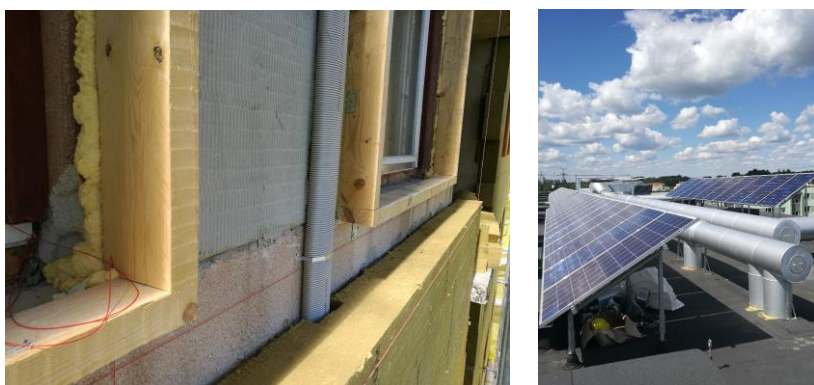
Figure 25. Ventilation pipelines in the external wall insulation, wooden frames to take windows in between the insulation layer (left) and PV panels (right).
