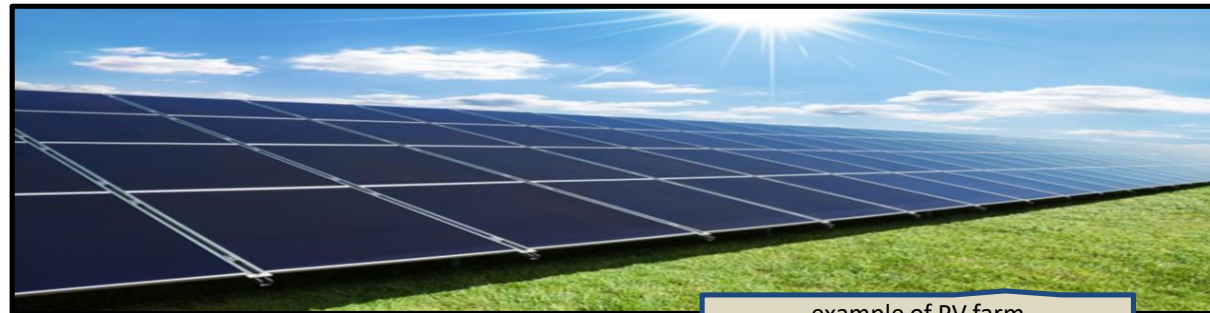
example of PV farm
