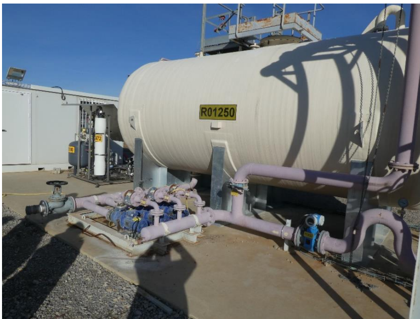
Figure 25. Discharge water collection tank
