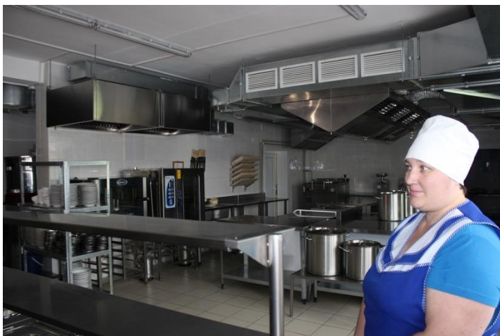
Energy efficient equipment in the kitchen, school № 4 in Dzerzhinsk, Minsk region
