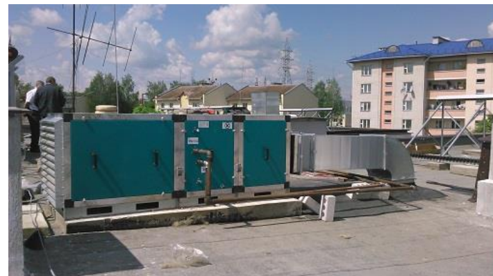
Waste heat recovery in kindergarten № 6 in Oshmiany, Grodno region
