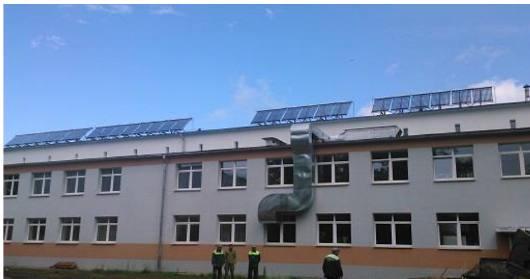
Solar collectors in machinery college in Vitebsk
