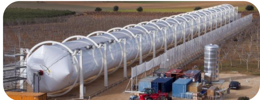
Industrial application in Spain (2016)
