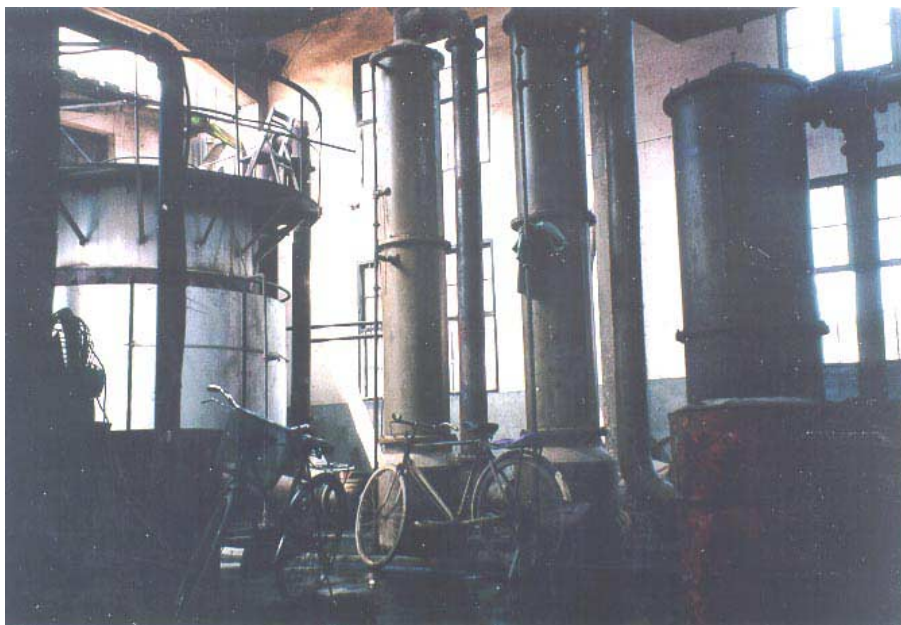
Figure 10 Open core downdraft gasifier running on rice husks with gas scrubbers
