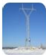
High voltage network
