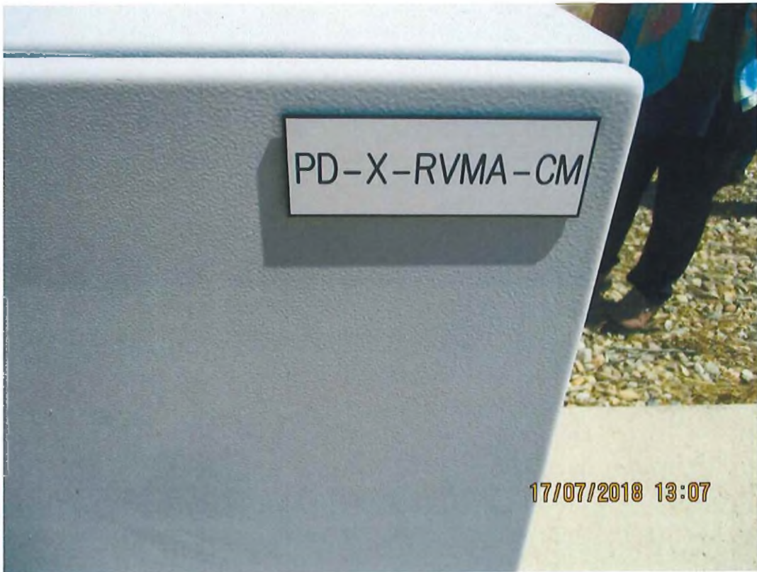
Figure 5: Emergency dose rate monitor
