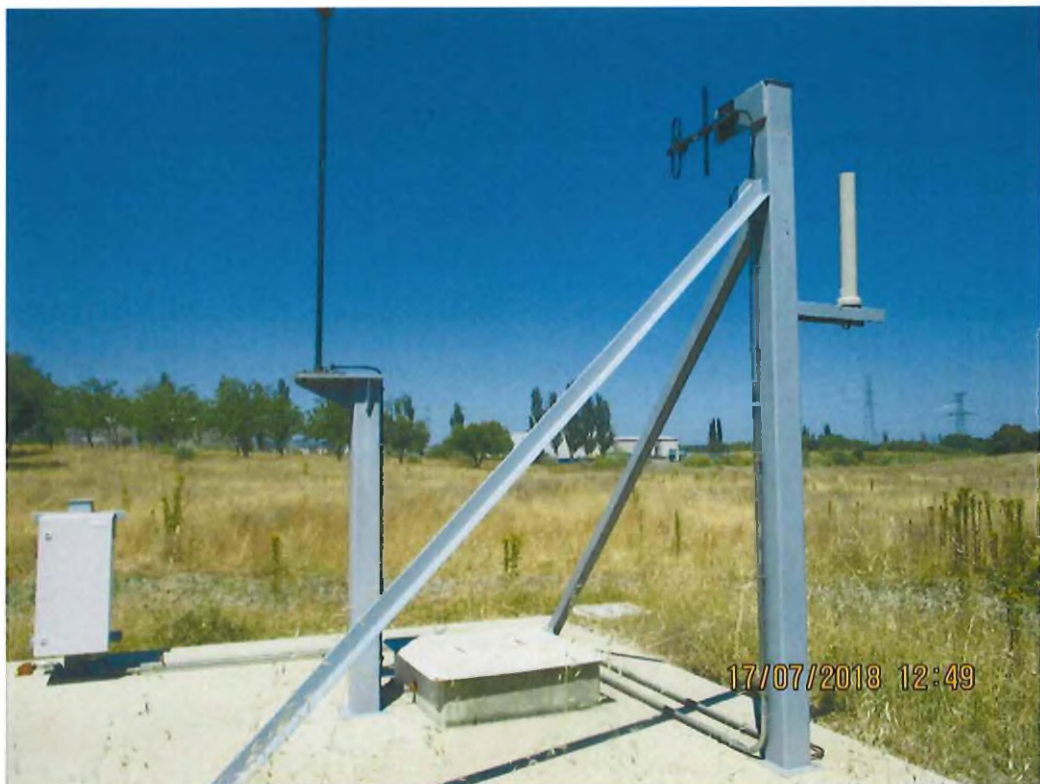
Figure 3: Emergency dose rate monitor
