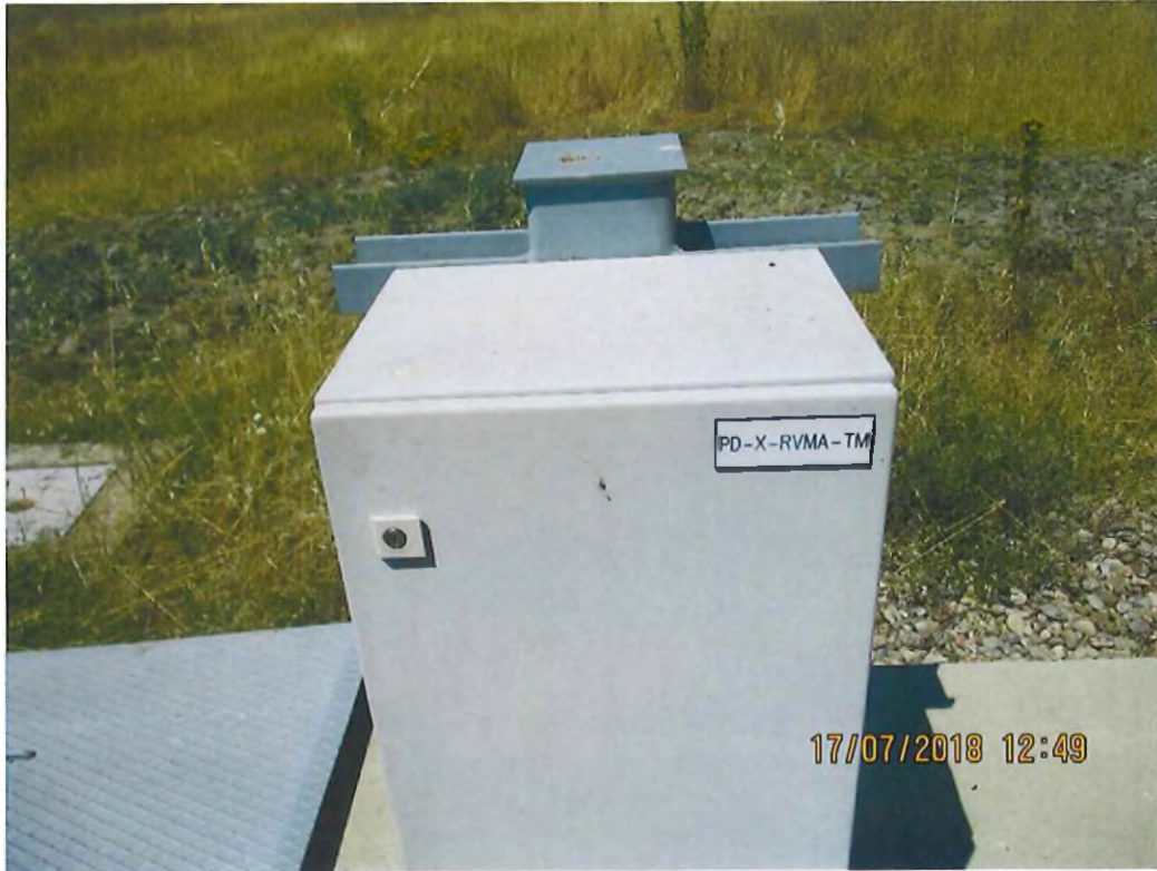
Figure 4: Emergency dose rate monitor
