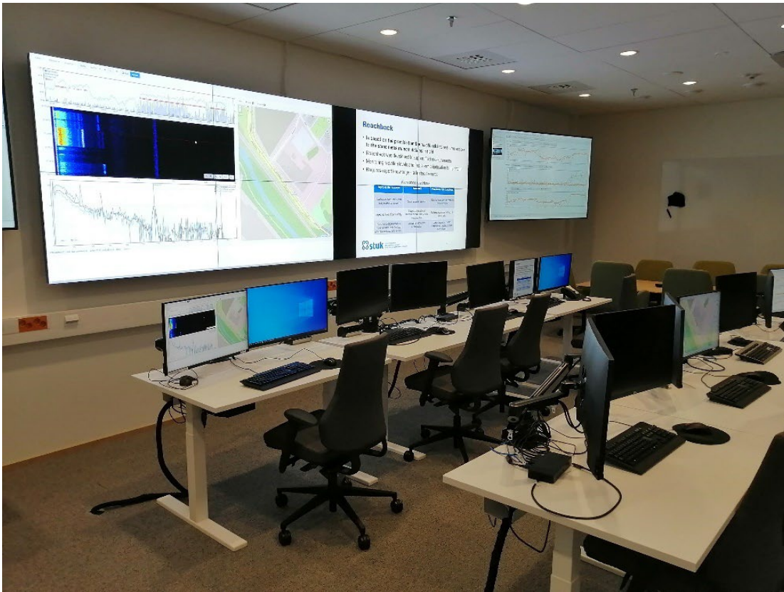
Figure 12. 'Reachback' environmental monitoring support facility at STUK
