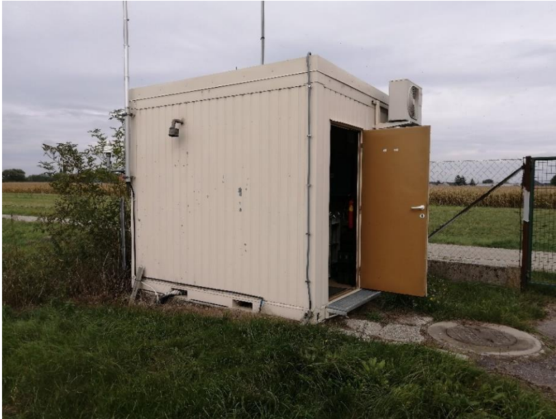
Figure 17. BITT AMS02 radiological monitoring container
