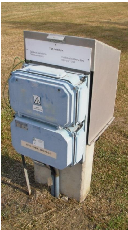
Figure 14. Teledosimetric station TDS inside the fence
