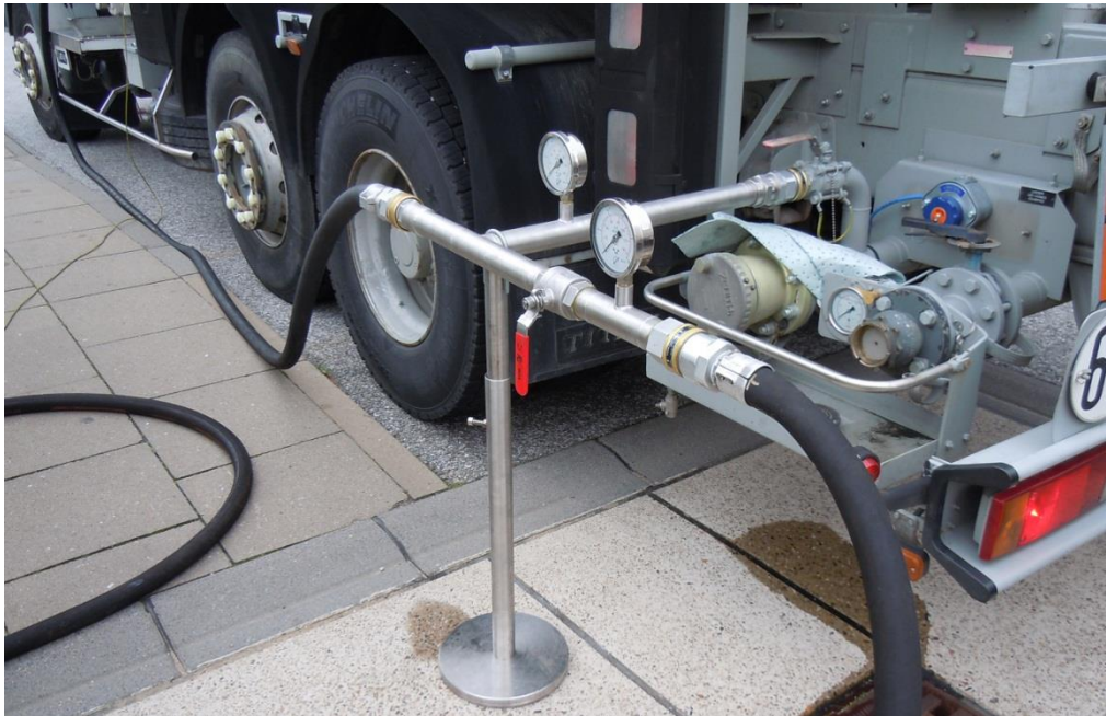
Figure 48: Fuel Truck piping arrangement
